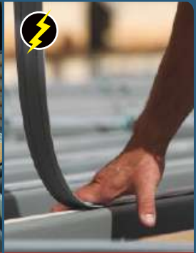
The installers applied bond then laid the track down onto the glue.
