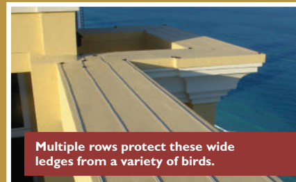
Two rows protect these sills. Notice the thin wire that connects the tracks at the next window.
